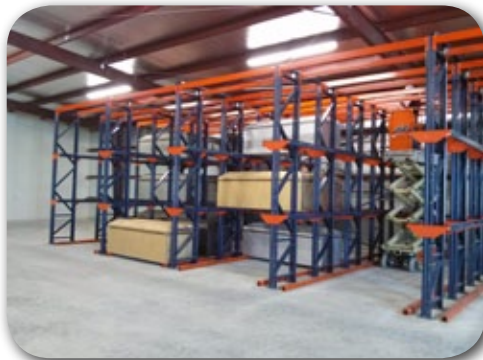
Mecalux Interlake racks just installed Baton Rouge, LA
